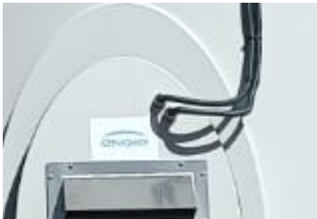
Illustration 8: Wiring through WTG door
