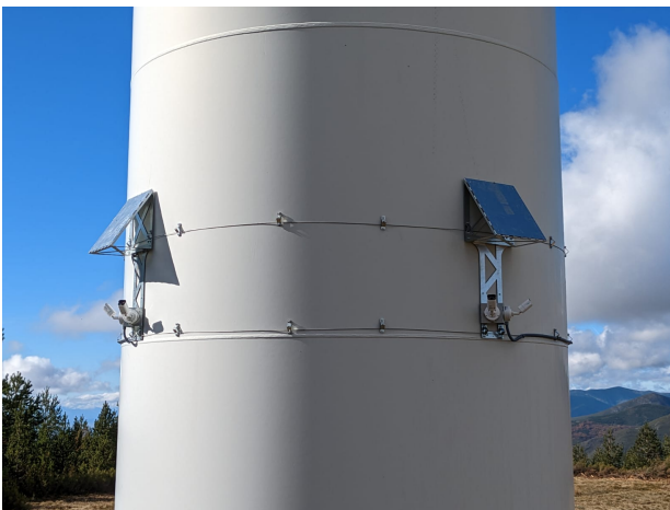
Figure 8: Camera Installation Example
