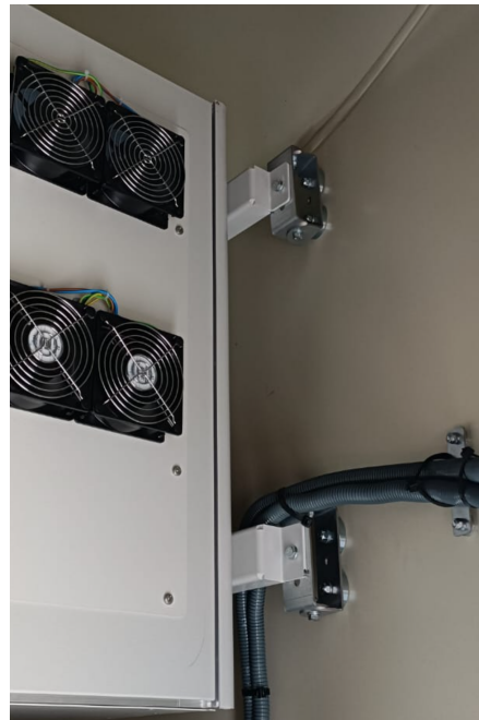
Illustration 2: Magnets used to secure the rack in the WTG
