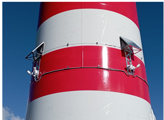
Figure 9: Camera Installation Example
