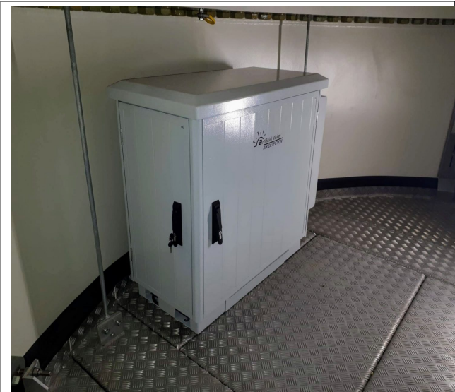
Illustration 6: ArtificialVision U-Detection installed in WTG's first floor
