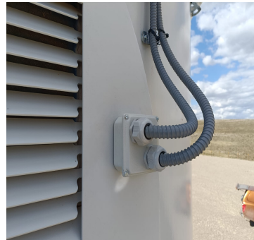
Illustration 9: Wiring through WTG door
